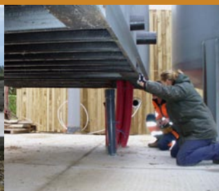
piping: levering pomphuis
